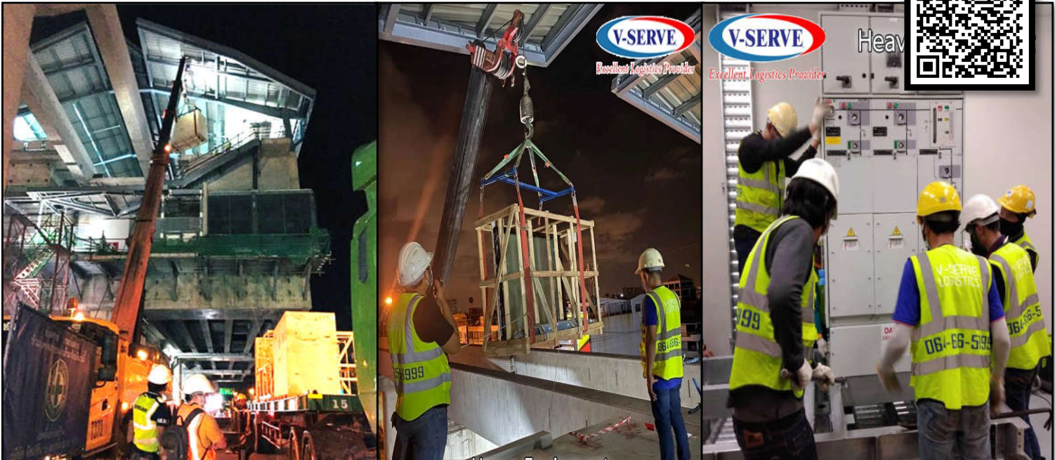
Installation of Electrical Equipment and Sky Train Barriers in 2020/21, approximately more than 80 stations
